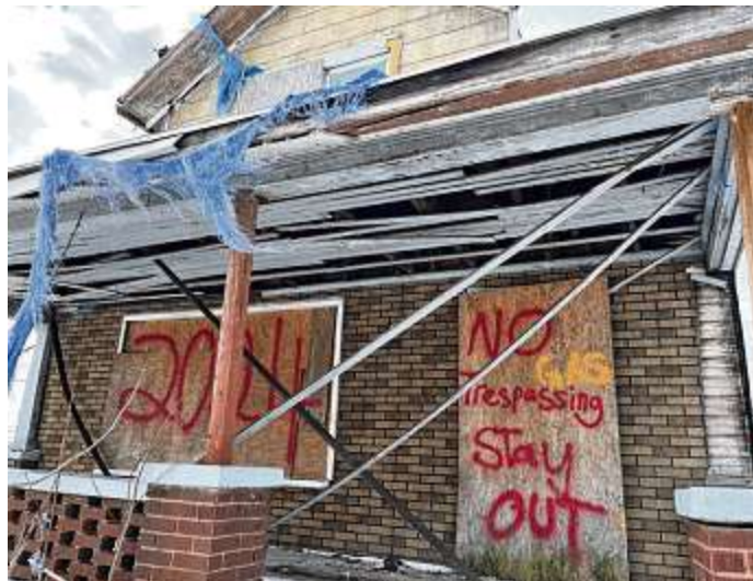
A vacant, abandoned and “dangerous” residential structure in Harrison Twp. that the township planned to demolish.
