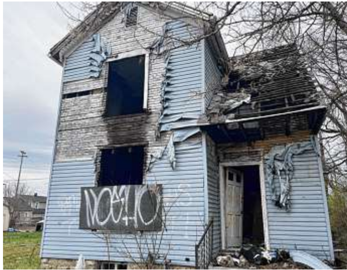
An abandoned home in East Dayton is among the structures that could soon be demolished.
